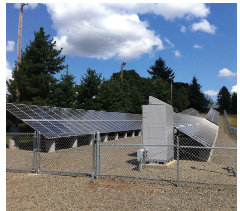
The BLM district office in Salem, Oregon showcases the agency's commitment to renewable energy with this ground-mounted 100 kW photovoltaic field.
