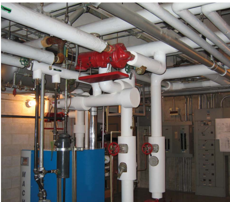
An investment in new boilers at the National Interagency Fire Center in Boise, Idaho provides energy efficiency for decades to come.
